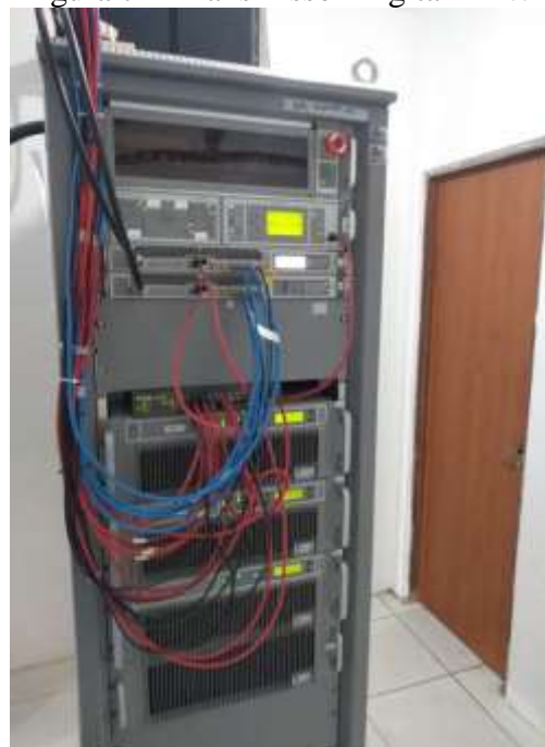
Figura 7 – Transmissor Digital 2 kW
